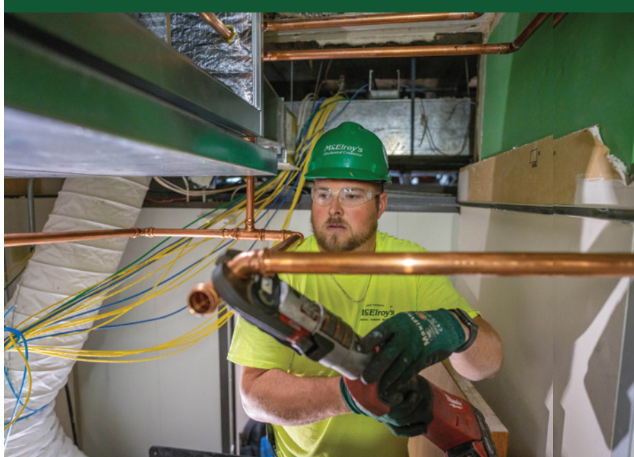
Top to bottom: A McElroy's journeyman plumber carefully measures and laser-aligns piping systems for precise craftsmanship Plumbing technician uses a ProPress crimping tool to join copper pipe securely, without heat Brazing copper pipe in the domestic water supply lines of the new Washburn University Law building
